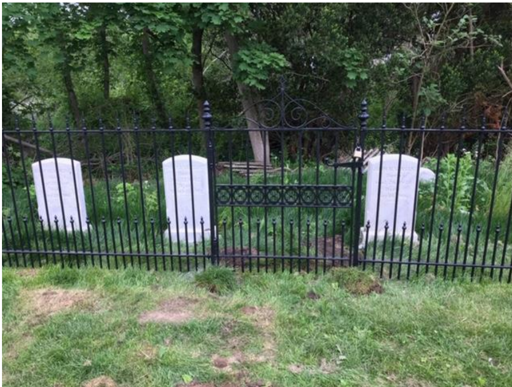
Restored historic iron fence and cleaned and reset headstones at Millington burial ground.
